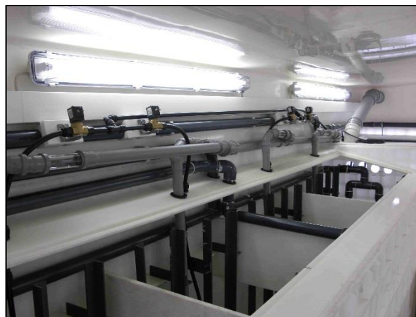
Inside of the polyethylene module – MBR stage
