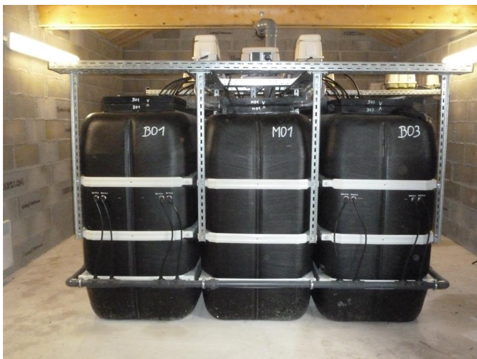
BUSSE-MF system consisting of 4 tanks á 3.600 l volume.
