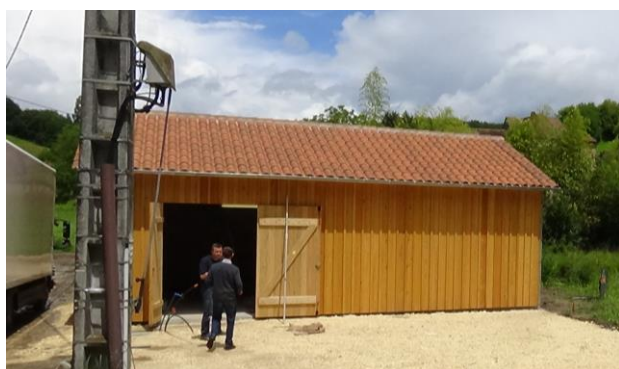
BUSSE-MF installed in a building that has been erected for the treatment system.
